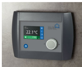
Solar Control Panel
